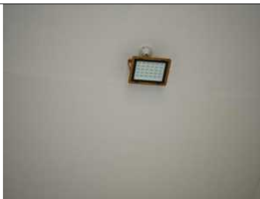
危废间防爆灯
