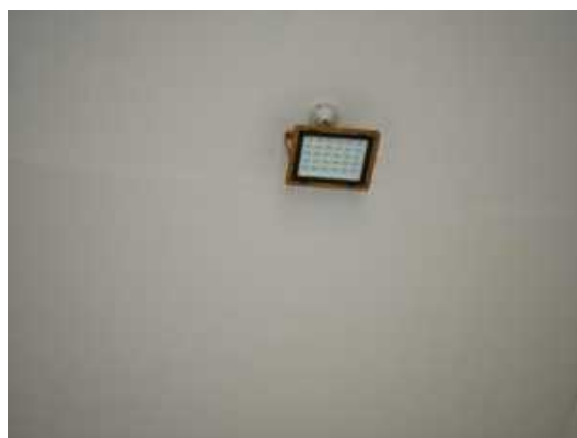
危废间防爆灯
