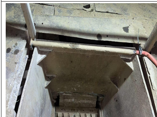
破碎机入料口喷淋
