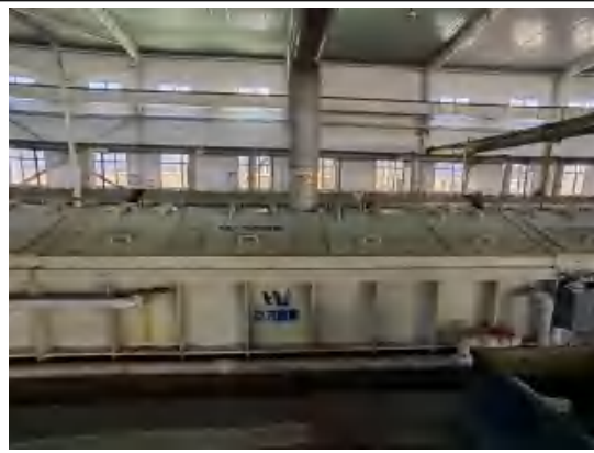
碱洗后水洗槽
