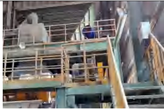
筛分车间内雾炮-2
