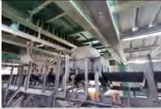
转运站转运点集气罩+喷淋
