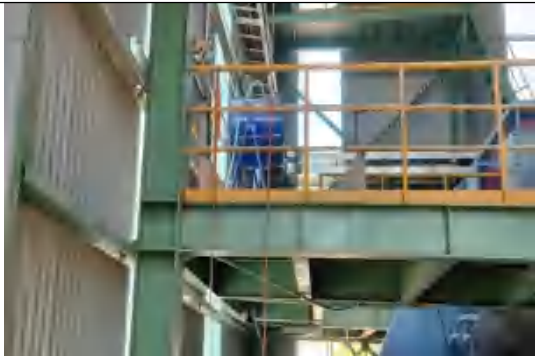
粗破车间内雾炮-1
