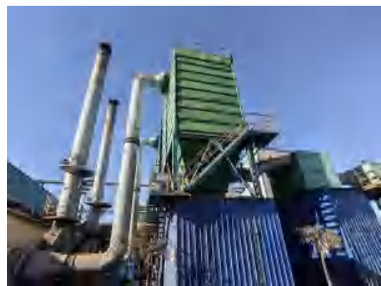
2#回转窑多管除尘器+脉冲布袋除尘器 +25m 排气筒[P2]
